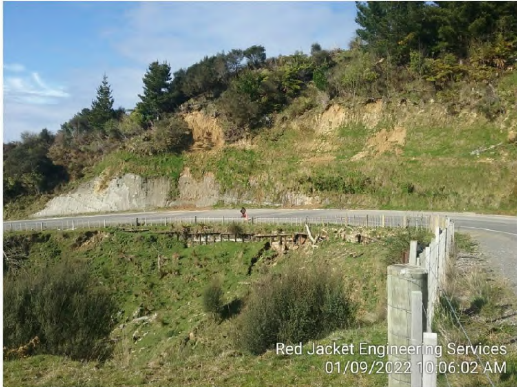
Figure 3 – Mangaotuku Rd retaining wall. Some of this wall will be repaired as well as the worst sections being replaced.
