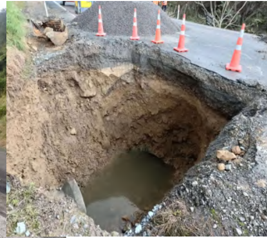
Culvert washout at Awakino 3 May
