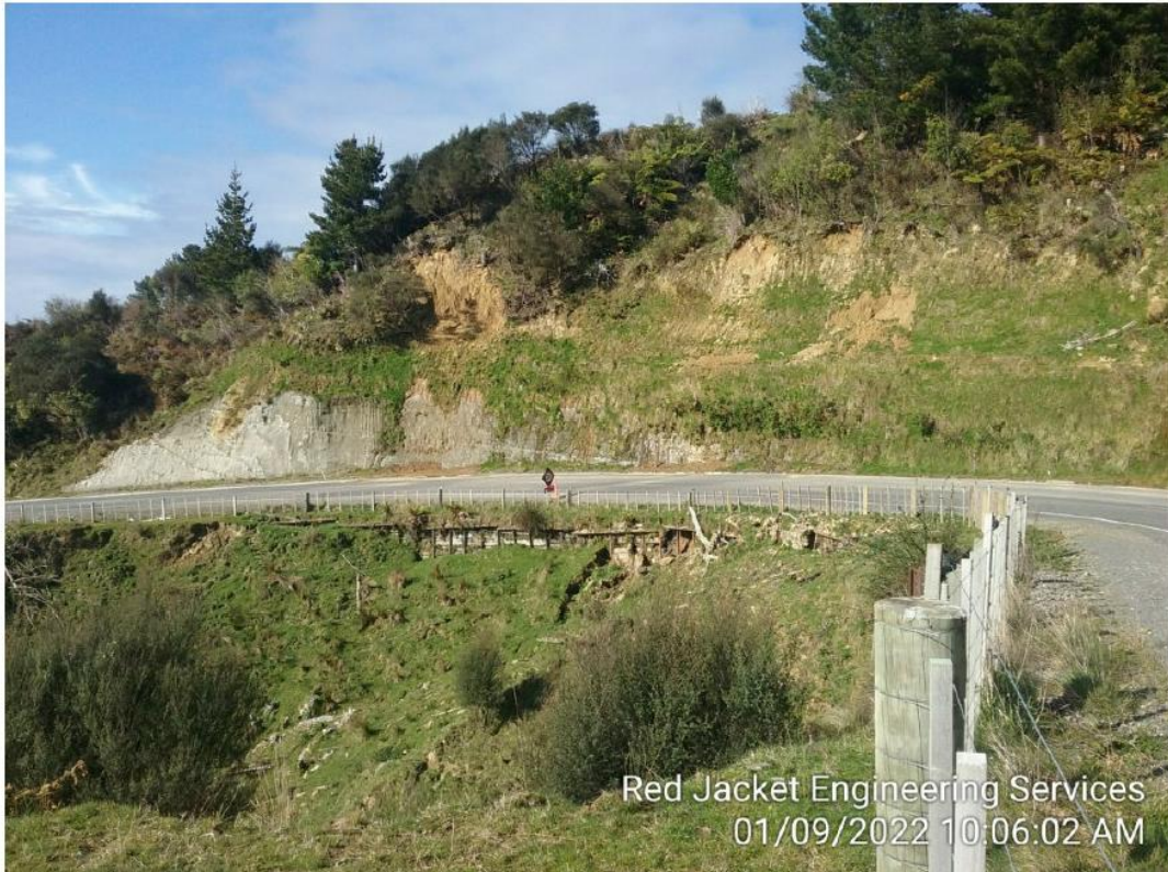
Figure 3 – Mangaotuku Rd retaining wall. Some of this wall will be repaired as well as the worst sections being replaced.
