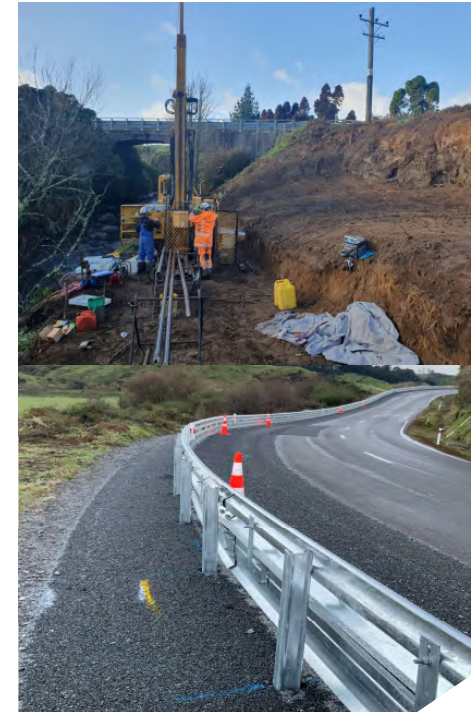
Top image: Proof drilling at Kahouri Stream Bridge Bottom image: New guardrail with motorcycle protection installed on SH43
