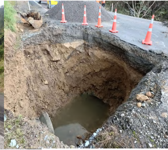
Culvert washout at Awakino 3 May
