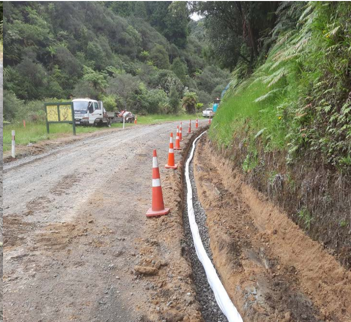
Prepared dish channel
