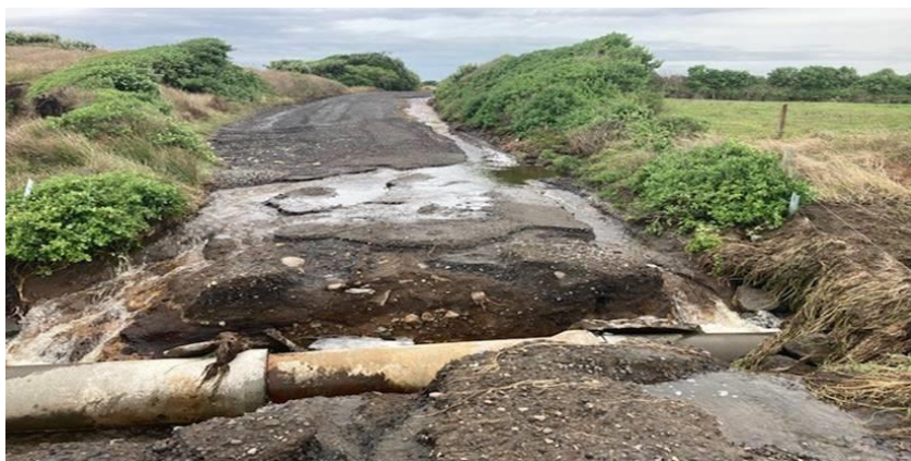
Stent Road Wash Out
