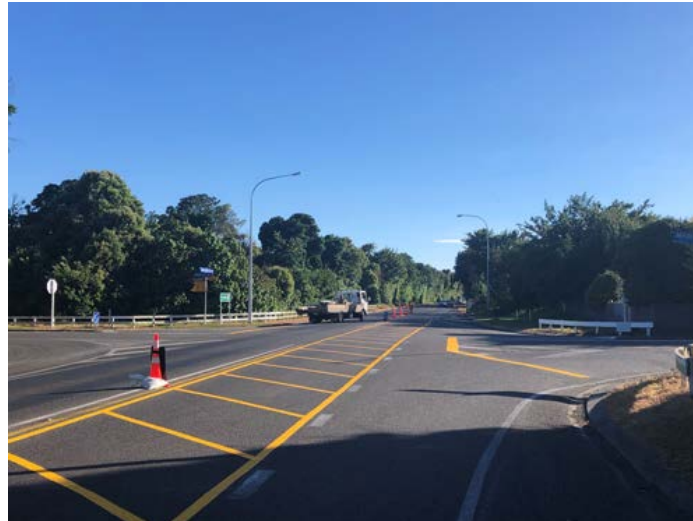
New line markings installed at the SH3/Princess street intersection to increase safety following feedback from local stakeholders and motorists
