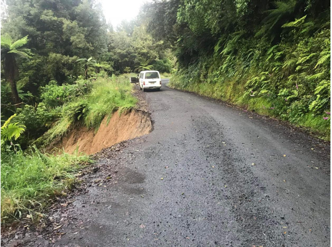
Figure 7 – Photo of the slip on Junction Rd approximately 1km from the Mangaopa Rd intersection.
