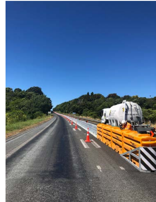
Concrete barriers installed to protect workers
