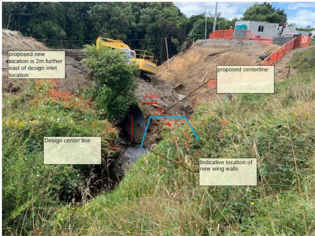
Figure 5 – Photo of the inlet of the existing steel culvert and the proposed location of the replacement culvert.
