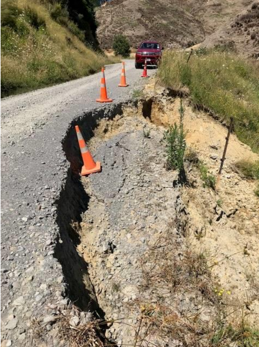
Figure 6 – Slip on Douglas North Rd
