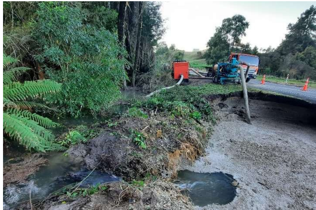
Water being pumped out of the collapsed culvert
