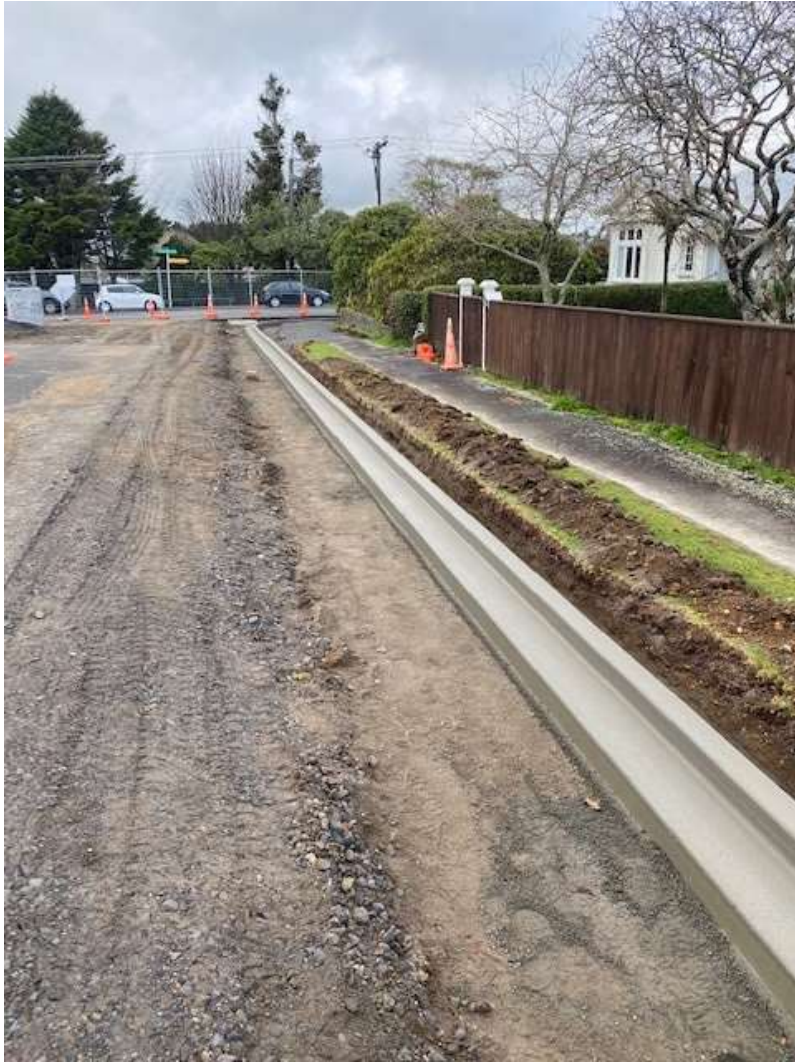
Figure 12 – Stratford High School Safety Project – Works in Progress showing the new extruded kerb and channel on Fenton Street.
