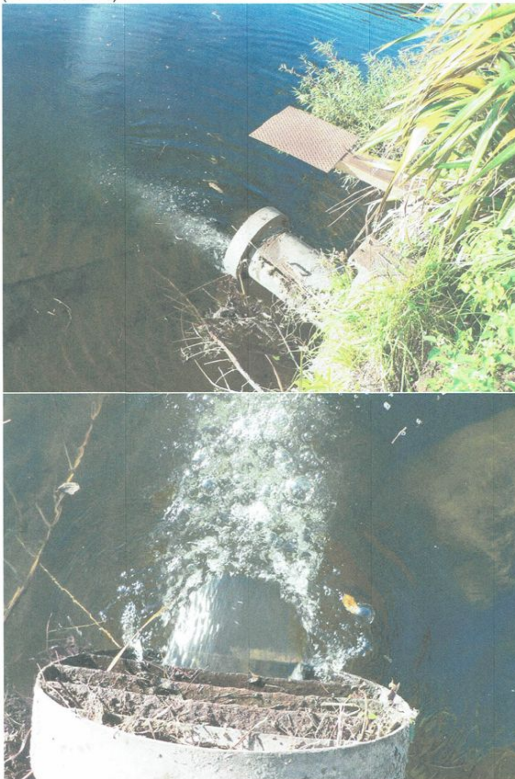
Lake Rotomanu intake – water flowing back out the inlet and into the Waiwhakaiho River (20 th March 2018)
