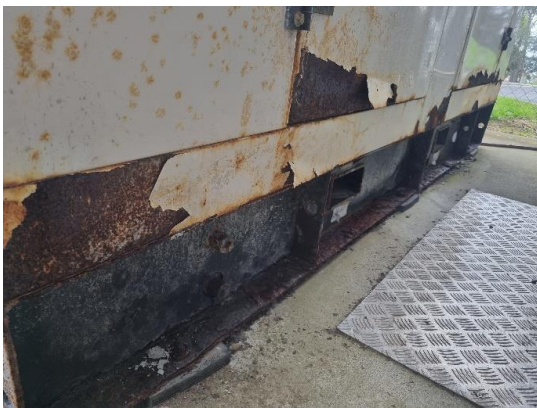
Photo 1 – Rust around frame
