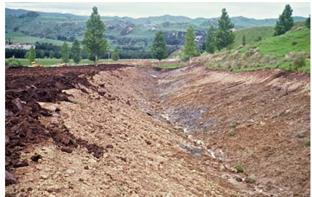
Figure 5. A shallow surface drain installed to remove excessive water away from the slip plane.
