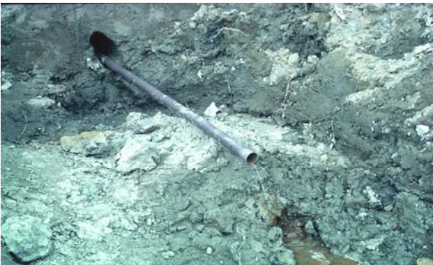
Figure 7. A pipe inserted into a horizontal bore for draining the slip plane.
