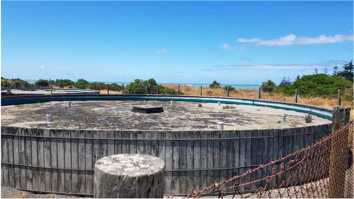
Photo 1 Sand filter beds comprising the Waiinu Beach Settlement wastewater treatment system (20 December 2017)
