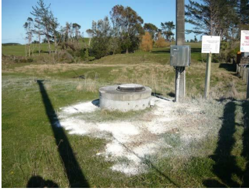
Photo 2 Inlet blockage and manhole overflow, September 2013
