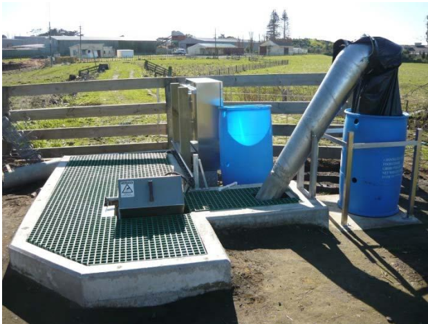
Photo 1 Step screen on the Waverley WWTP inlet
