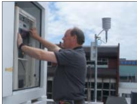
Figure 6 Thermo FH62 BAM monitor equipped with PM 10 SSI during installation by QEMS Ltd.
