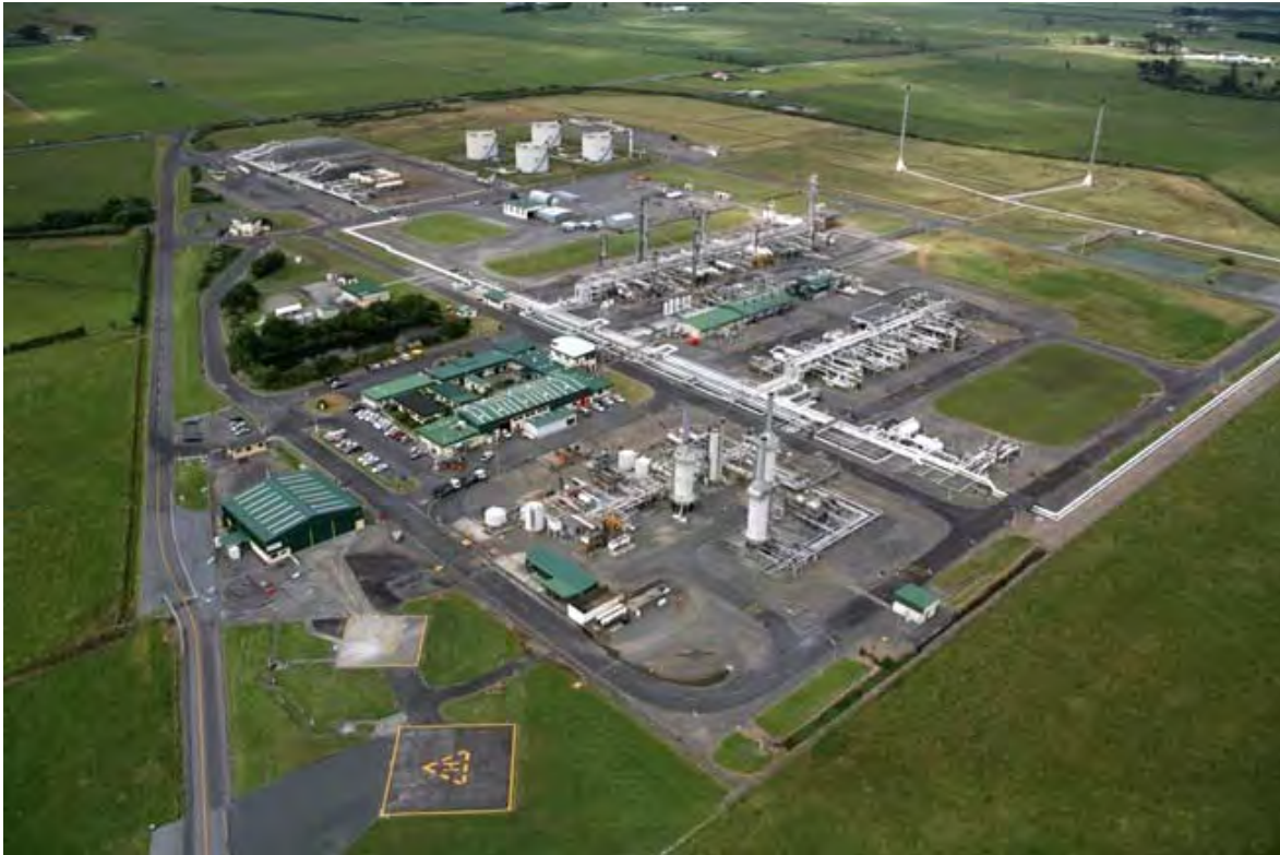
Photo 1 Maui Production Station
