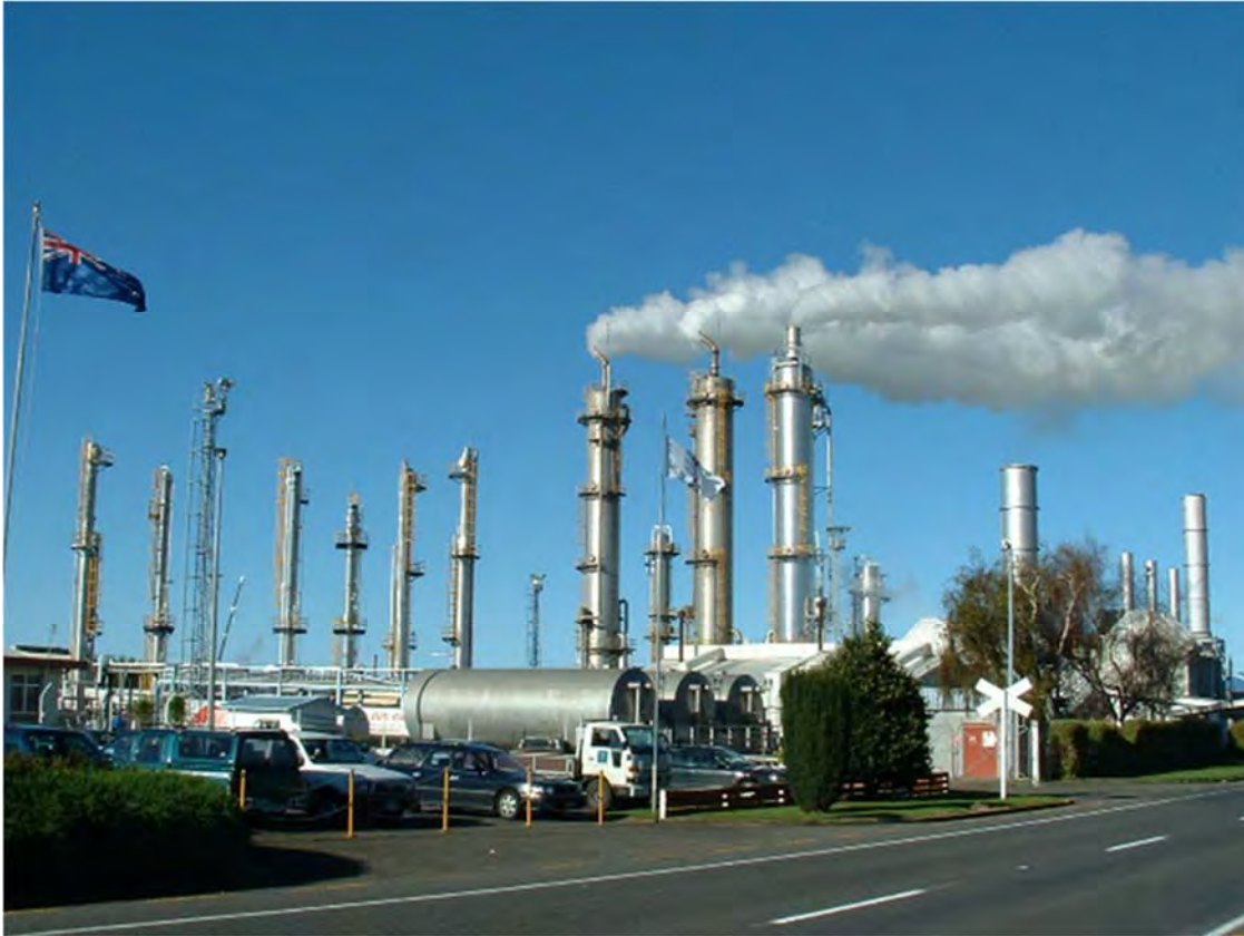
Photo 1 Vector KGTP during three train operation
