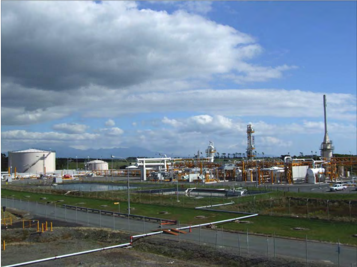
Photo 1 Pohokura Production Station
