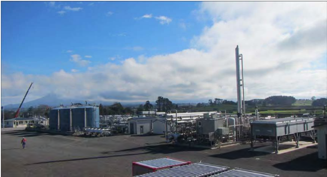
Photo 1 Cheal Production Station
