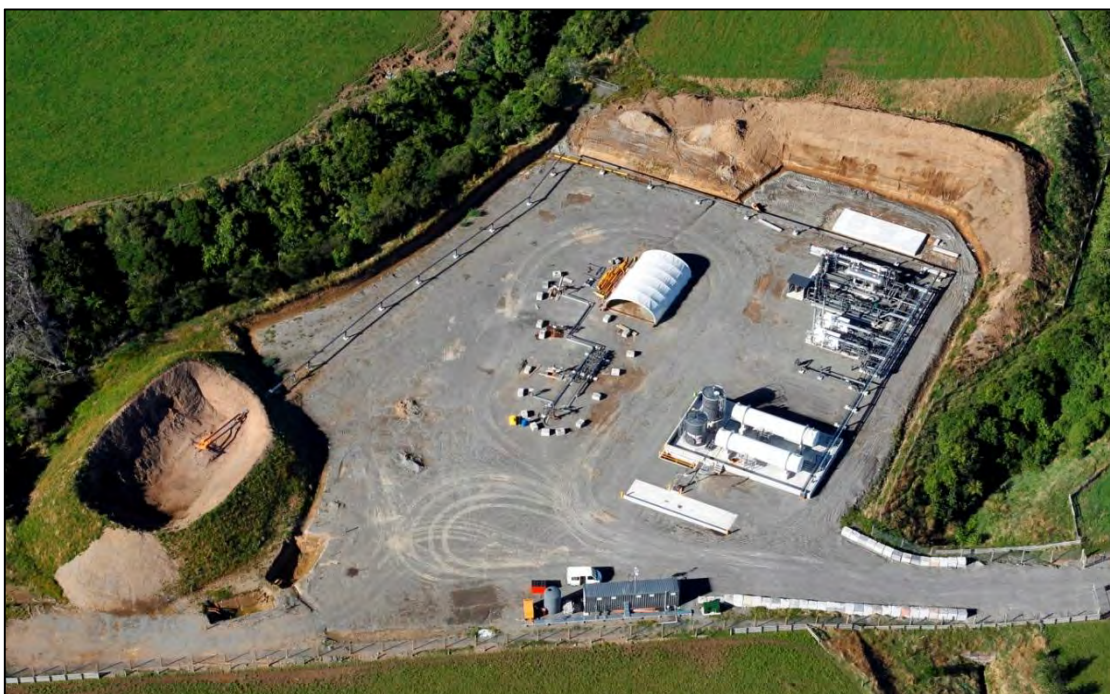
Photo 1 Sidewinder Production Station and wellsite in February 2012
