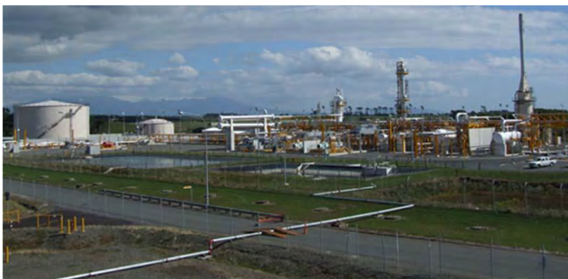
Photo 1 Pohokura Production Station
