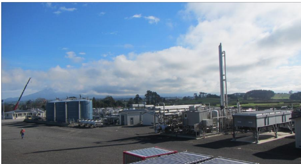
Photo 1 Cheal Production Station
