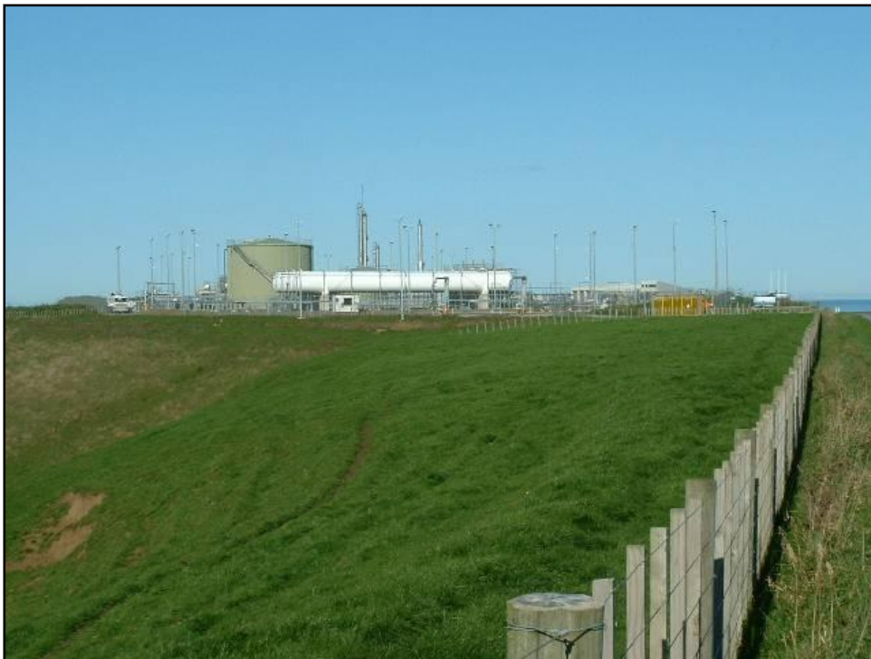
Photo 1 Rimu Production Station
