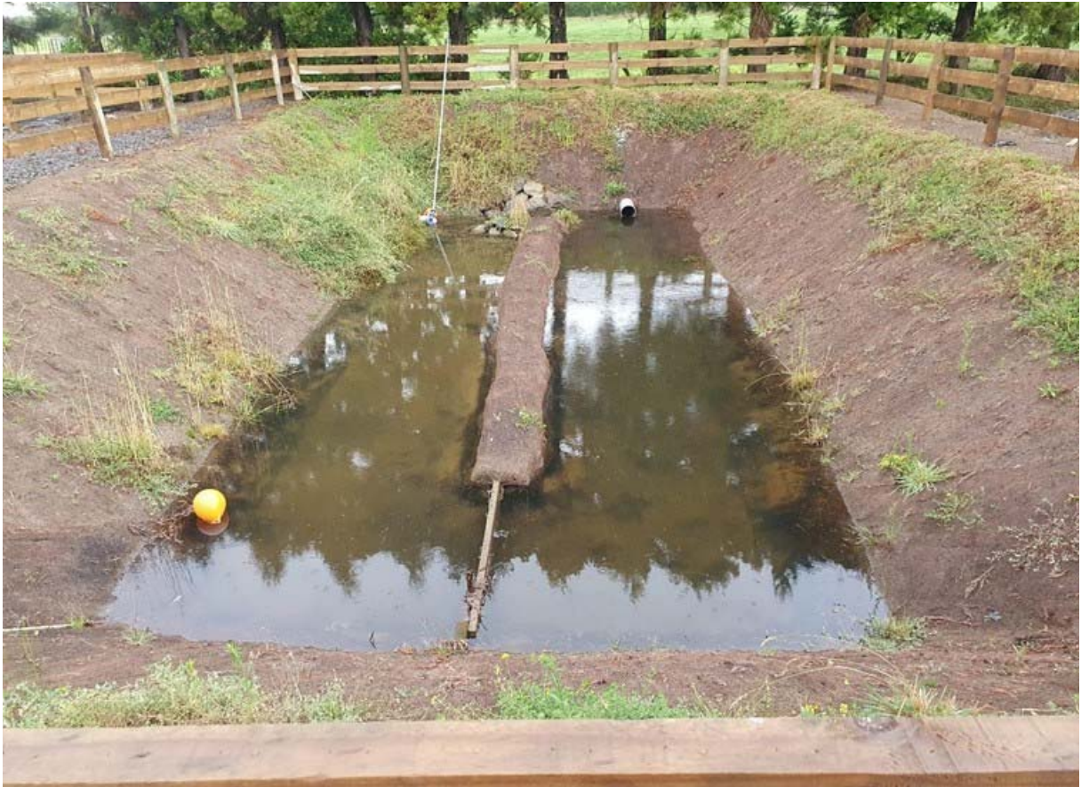
Photo 4 An additional unlined settling pond has been added in series with the existing two lined pits to further settle out suspended sediment prior to discharge
