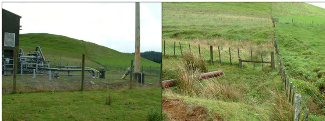
Photo 4 Ahuroa-B site looking towards the skimmer pit (left) and the final discharge point
