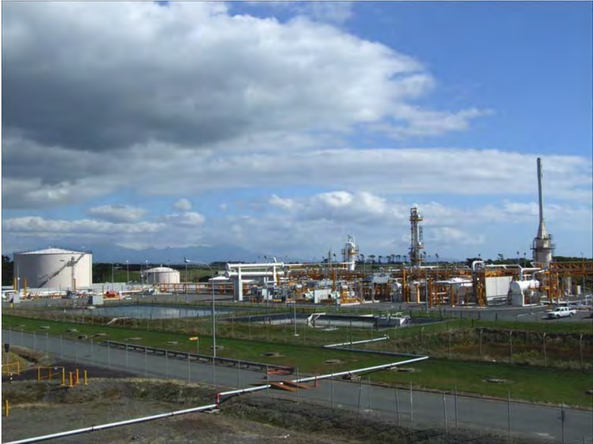
Photo 1 Pohokura Production Station
