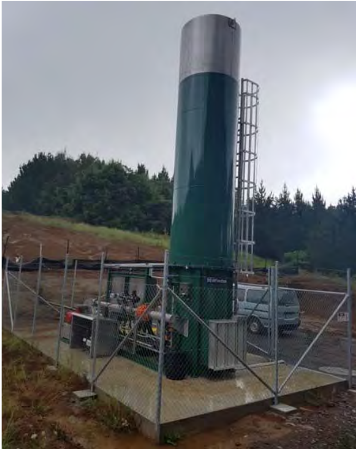
Photo 3 The fully enclosed flare
