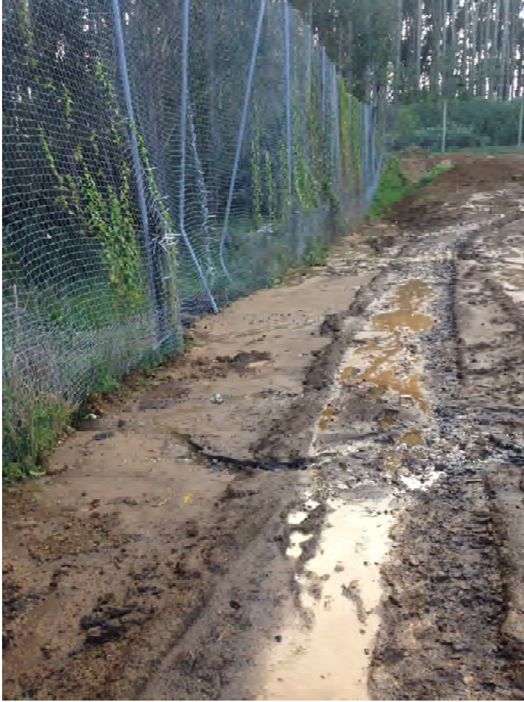
Figure 12 Silt between landfill northern batter and the leachate pond area, 23 May 2018
