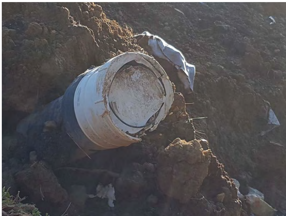
Photo 7 Broken leachate line cap, 11 July 2017
