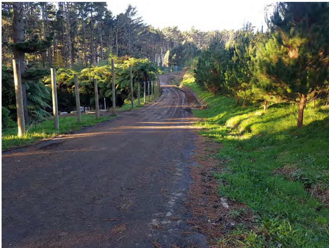
Photo 16 Silt on access road, 5 July 2017
