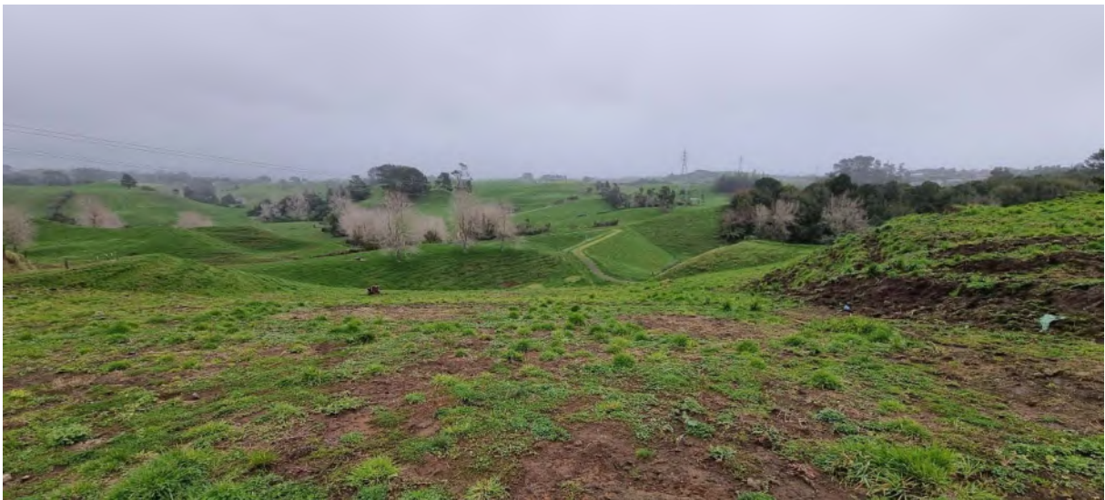
Photo 2 The state of the capping progress of the discontinued discharge site, as of 3 August 2022. Topsoil to be added on right hand side
