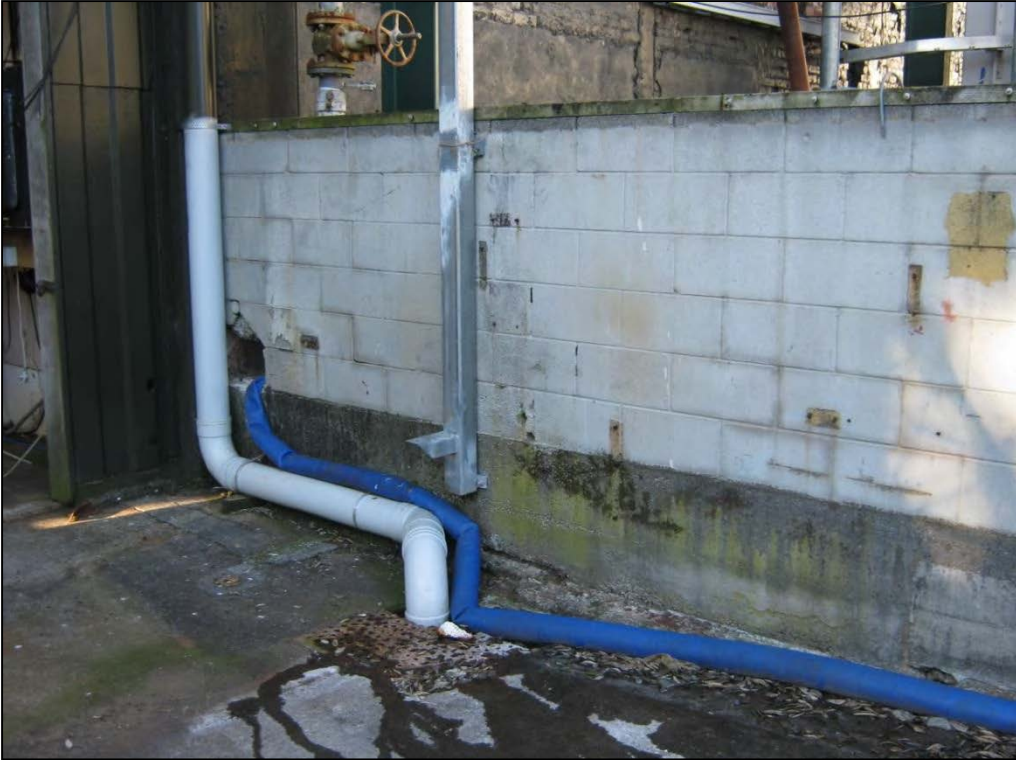
Photo 1 Oil cooling water sampling point at end of blue hose
