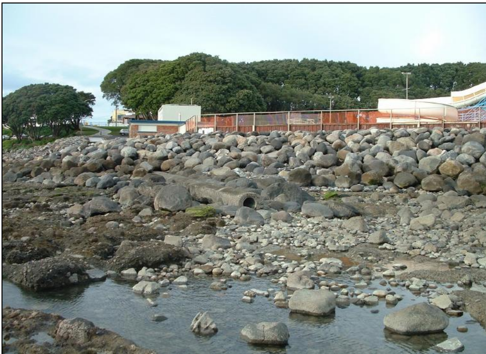
Photograph 1 Todd Energy Aquatic Centre ocean outfall
