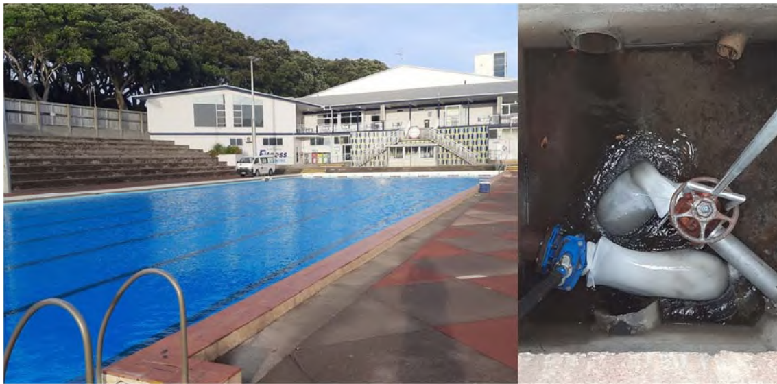
Photo 2 Todd Energy Aquatic Centre outdoor pool, and muslin cloths in place over outlet pipes (2 May 2023)
