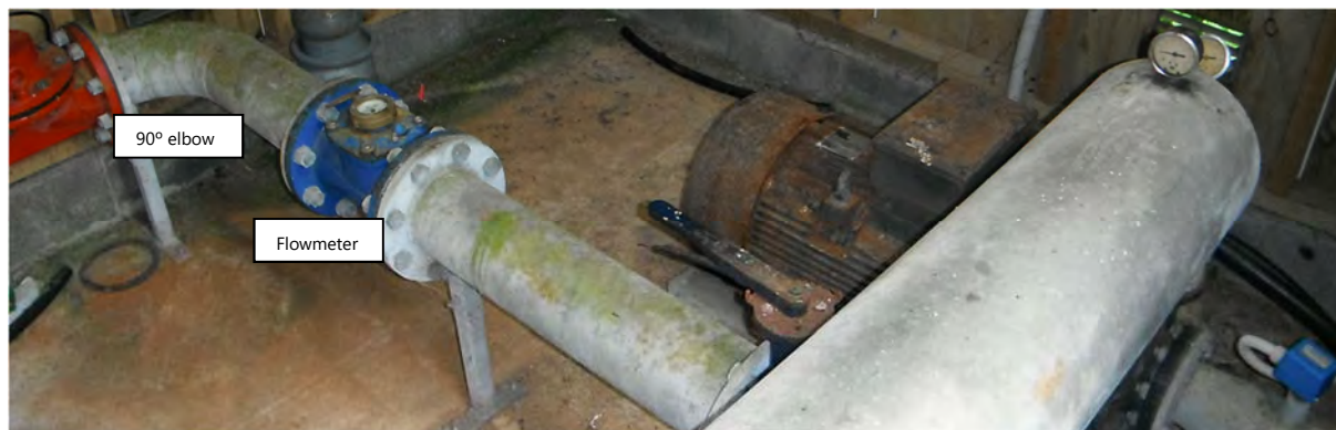
Photo 5 Poor installation of a flowmeter
