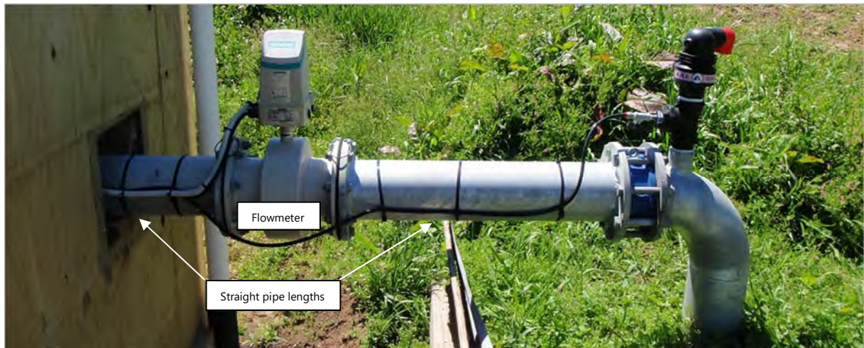
Photo 4 Good installation of a flowmeter
