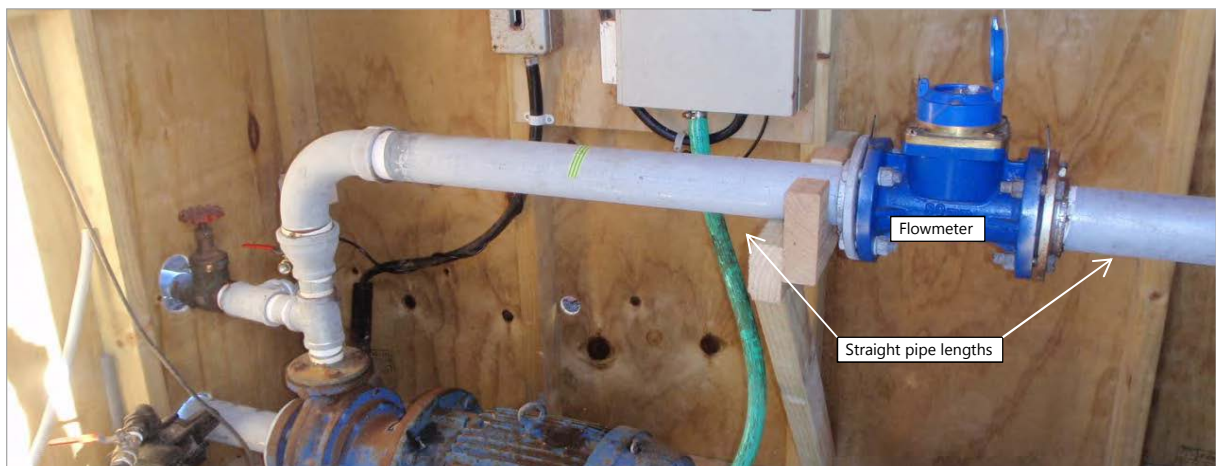
Photo 4 Good installation of a flowmeter
