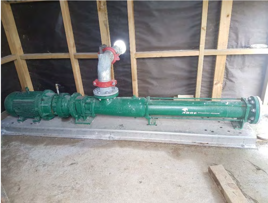
Figure 13 Inside the pump shed showing the multi stage variable speed pump
