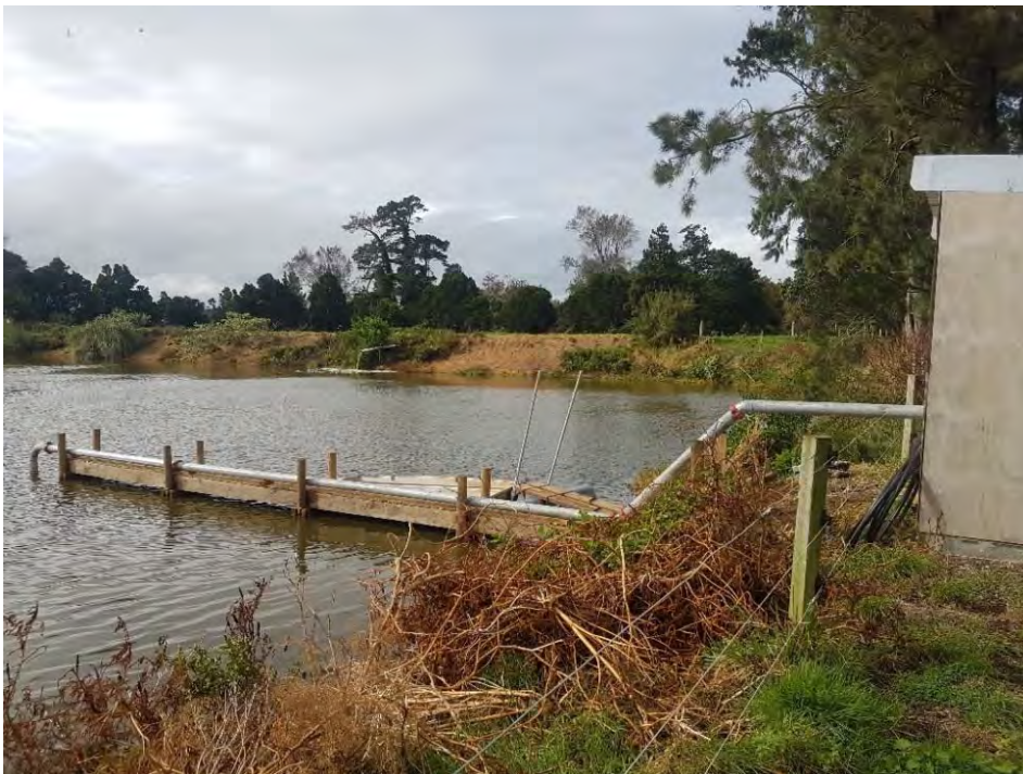
Figure 12 Pump systems from final aerobic ponds which transport effluent to the stream
