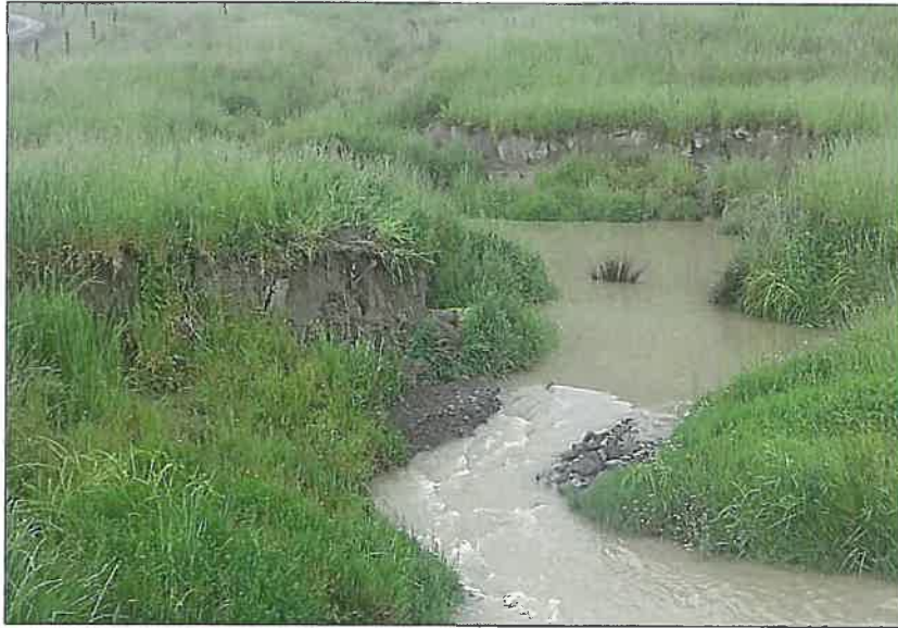
Photo 5 The outlet of the pool, directly below the main track access culverts, showing deposited gravels that are beginning to scour away
