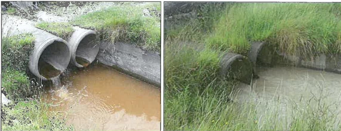
Photo 4 The access culvert immediately upstream of site 2, December 2015 (left) and December 2016 (right).
