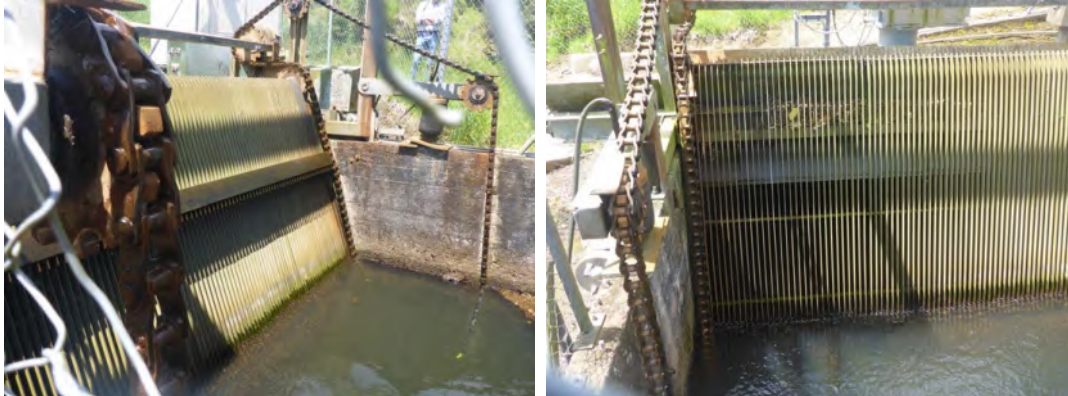
Figure 4.19. Trash screen at Lake Ratapiko intake to the Motukawa Power Station penstocks, February 2021.
