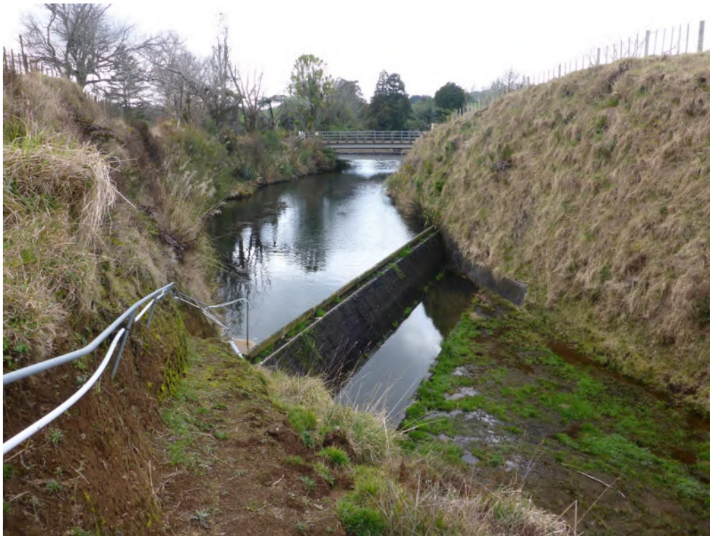
Figure 1.9. Lake Ratapiko spillway to Mako Stream, August 2019.
