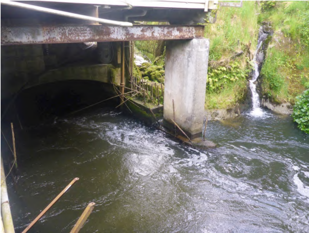
Figure 1.12. Motukawa Power Station tailrace (during generation), November 2018.
