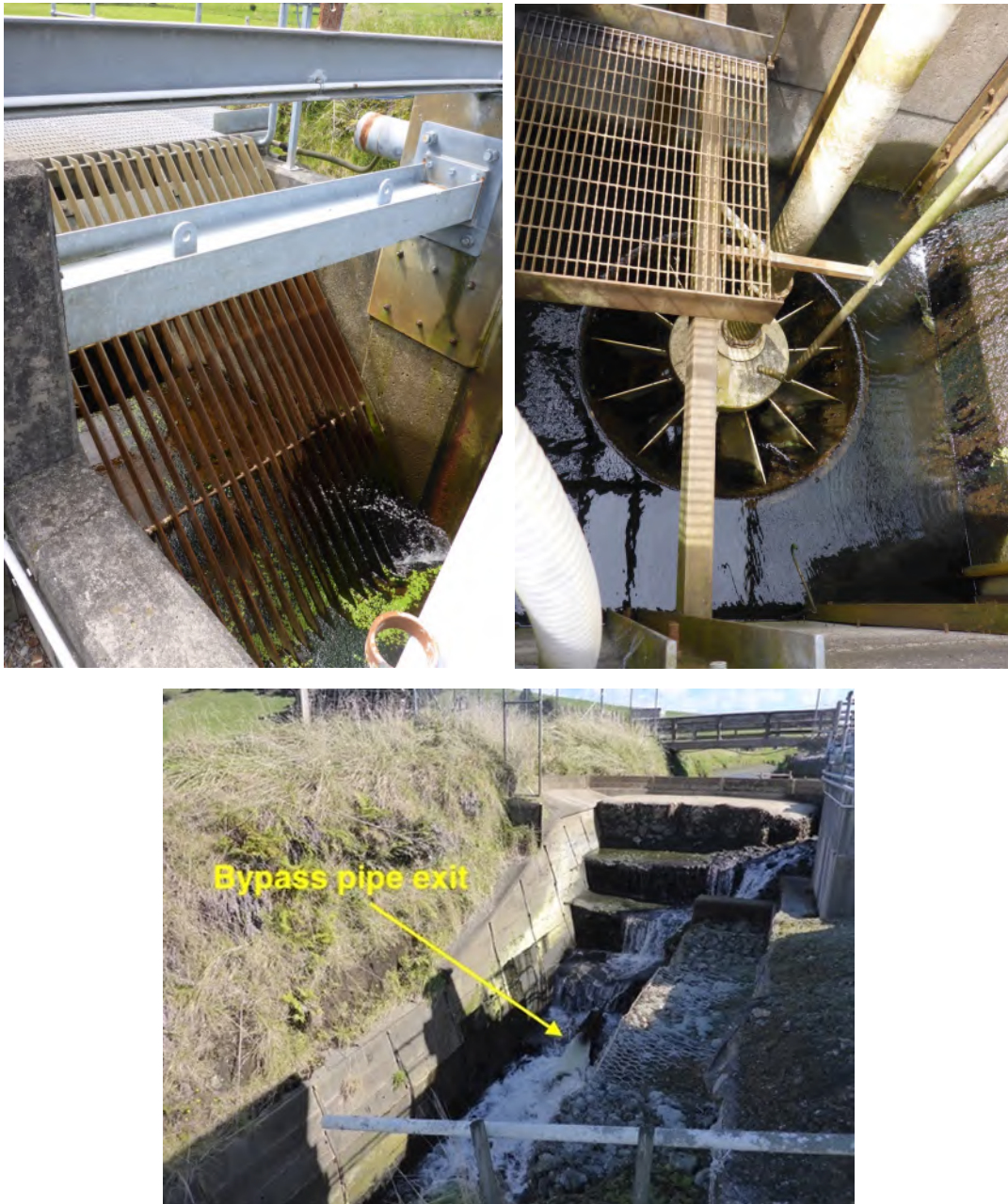
Figure 4.17. Top left: Trash screen on the Motukawa HEPS in-race generator. Top right: The Kaplan turbine. November 2018 (note, flow not being diverted and generator not operating). Bottom: Bypass pipe outlet at bottom of weir.
