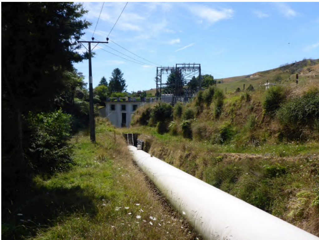
Figure 1.11. Penstock entering Motukawa Power Station, February 2020.
