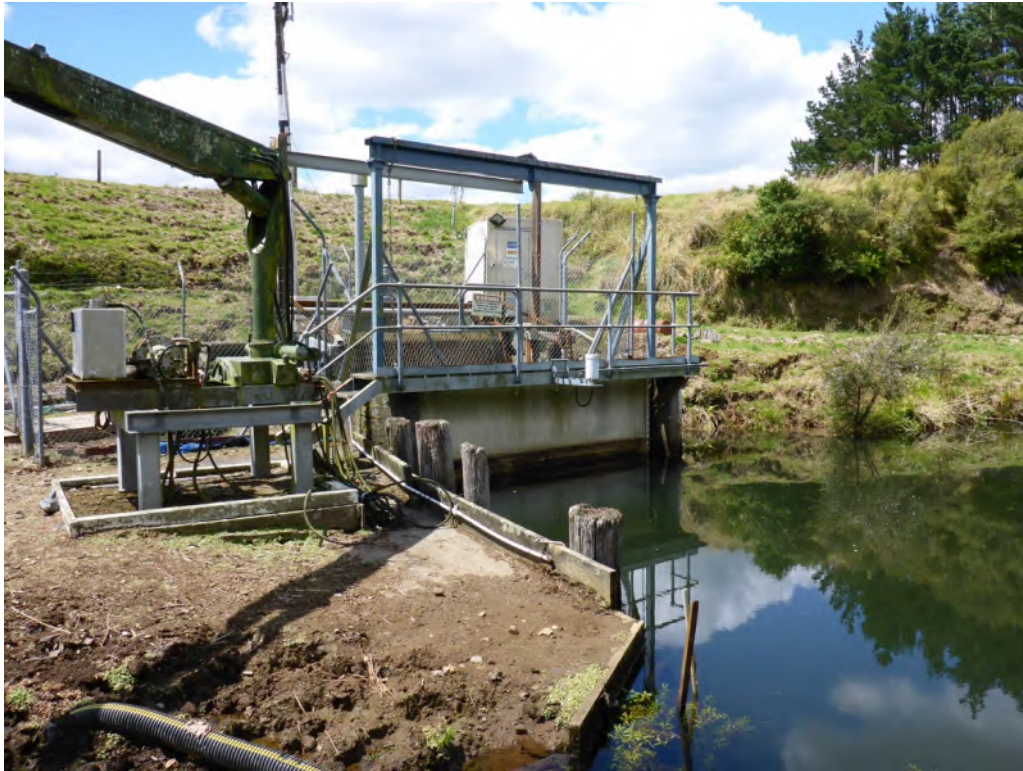
Figure 1.10. Motukawa HEPS intake to penstock at Lake Ratapiko, February 2021.
