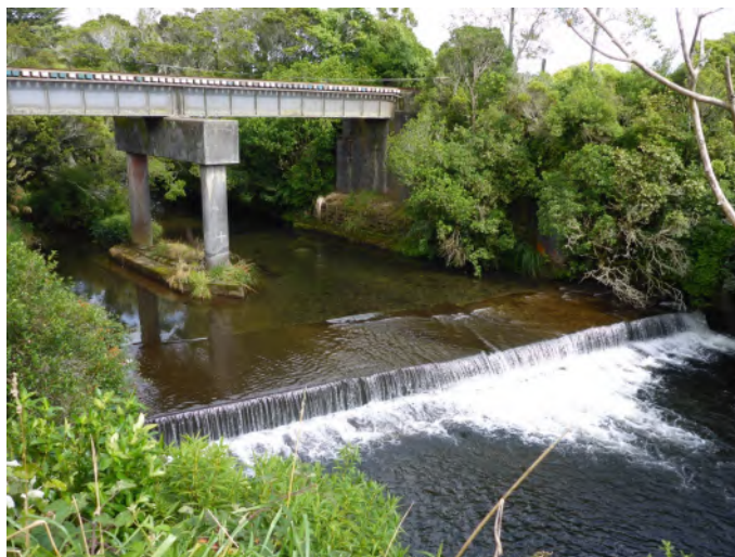
Figure 4.13. Weir in the Manganui River at SH3 near Midhurst, approximately 13 km upstream of the Motukawa HEPS intake weir, February 2021.
