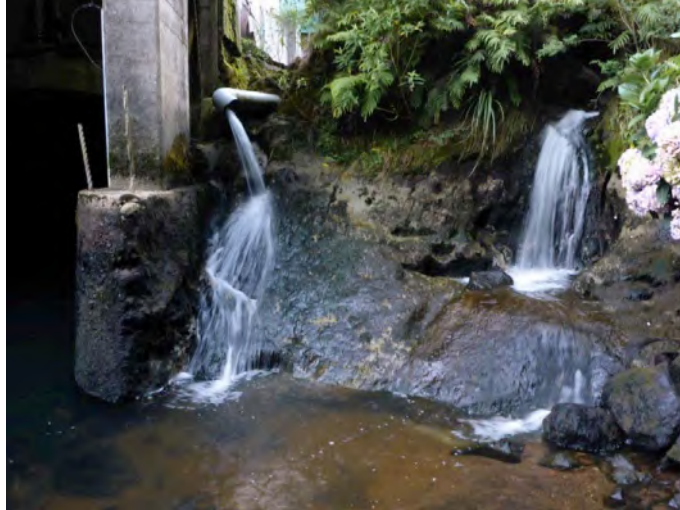
Figure 4.22. Watercourses entering from the true left of the Motukawa HEPS tailrace discharge, February 2021. The flow on the right of the photograph is from a natural watercourse. The flow on the left is piped.
