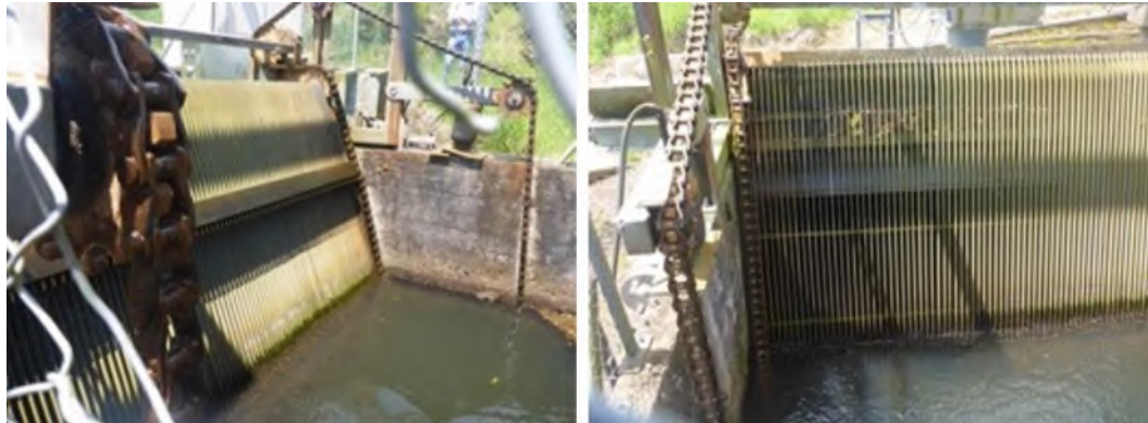
Figure 9: Trash Screen at Lake Ratapiko Power Station Intake
