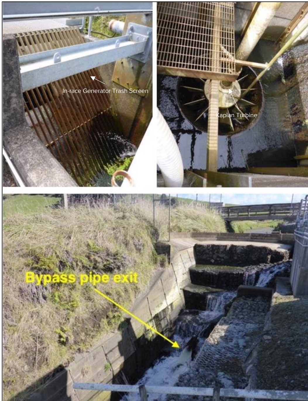
Figure 6: In-Race Generator Components
