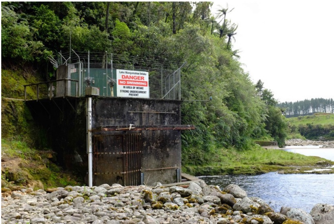
Figure 1.3. Mangorei HEPS intake structure on the Waiwhakaiho River.
