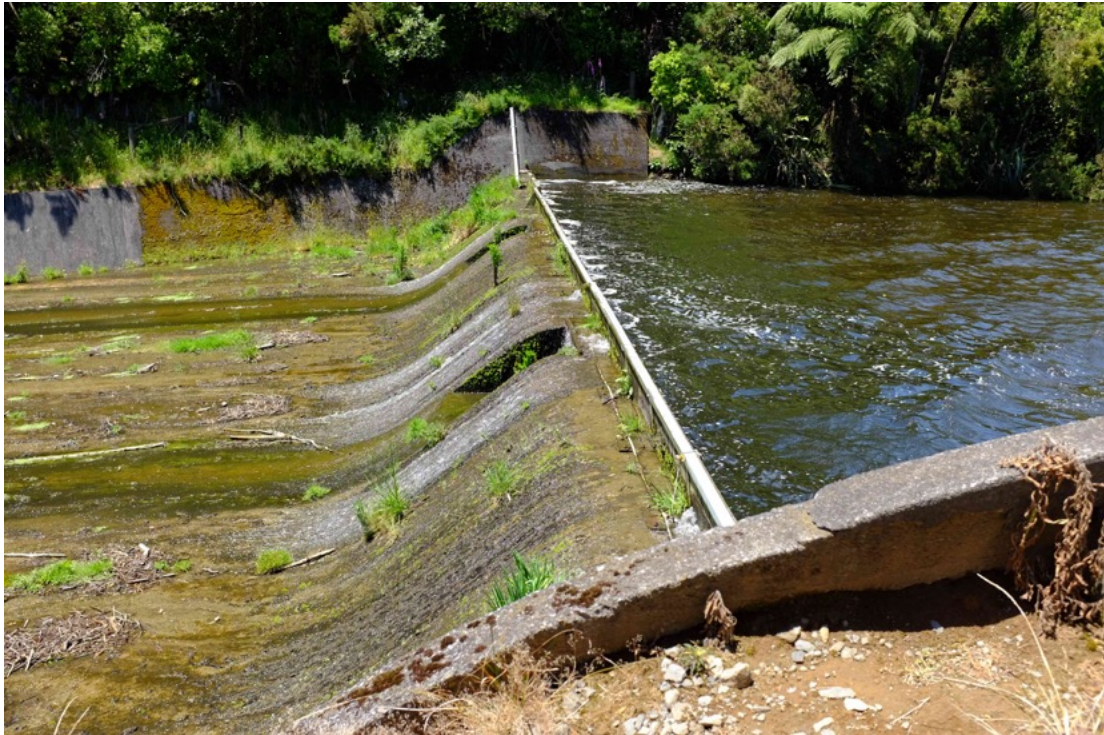
Figure 1.6. Standing on the Lake Mangamahoe earth dam looking across the concrete spillway.
