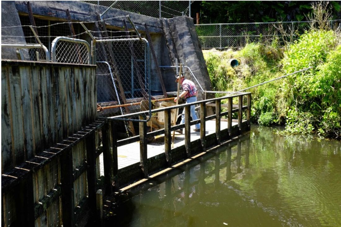
Figure 1.8. Mangorei HEPS intake to penstocks at Lake Mangamahoe.
