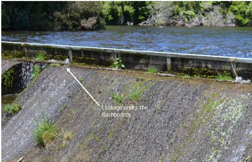
Figure 3.10 Tipping flashboards mounted on the crest of the concrete spillweir at Mangamahoe Dam. Note the discrete leakage points at the interface between the flashboards and the concrete weir
