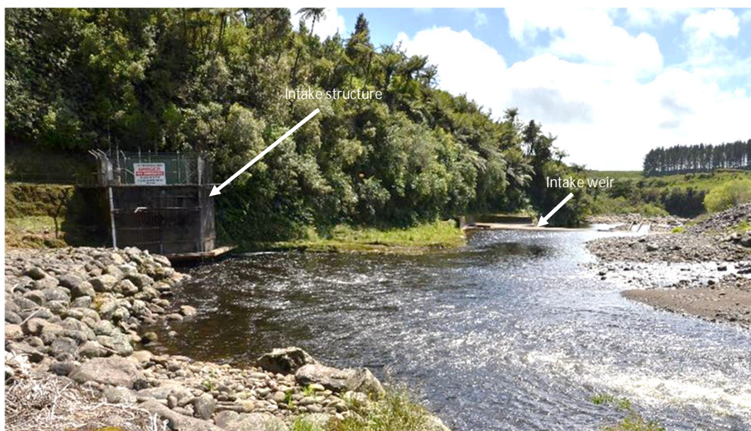
Figure 3.3 Intake structure on left bank of Waiwhakaiho River (photo taken looking downstream)
