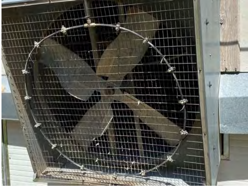
Photo 7 Sidewall fan mister configuration
