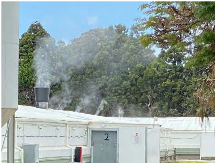
Photo 6 New ridgeline fan on Shed 2; roof fan and endwall misters in operation
