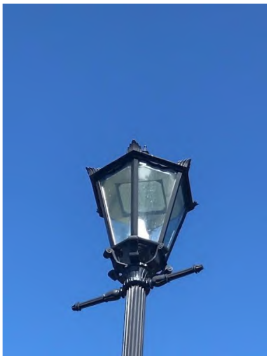
Streetlight in Mercade Close.
