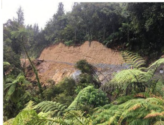
Safety Improvement on Junction Road where a logging truck rolled over down the bank on a narrow section of the road.
