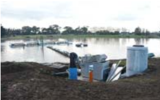
Photo 3 Step screen at new inlet to primary pond, June 2009
