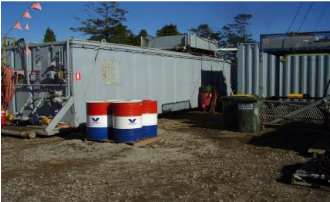
Photo 2 The bulk fuel, water tank and smaller fuel tank above the water tank
