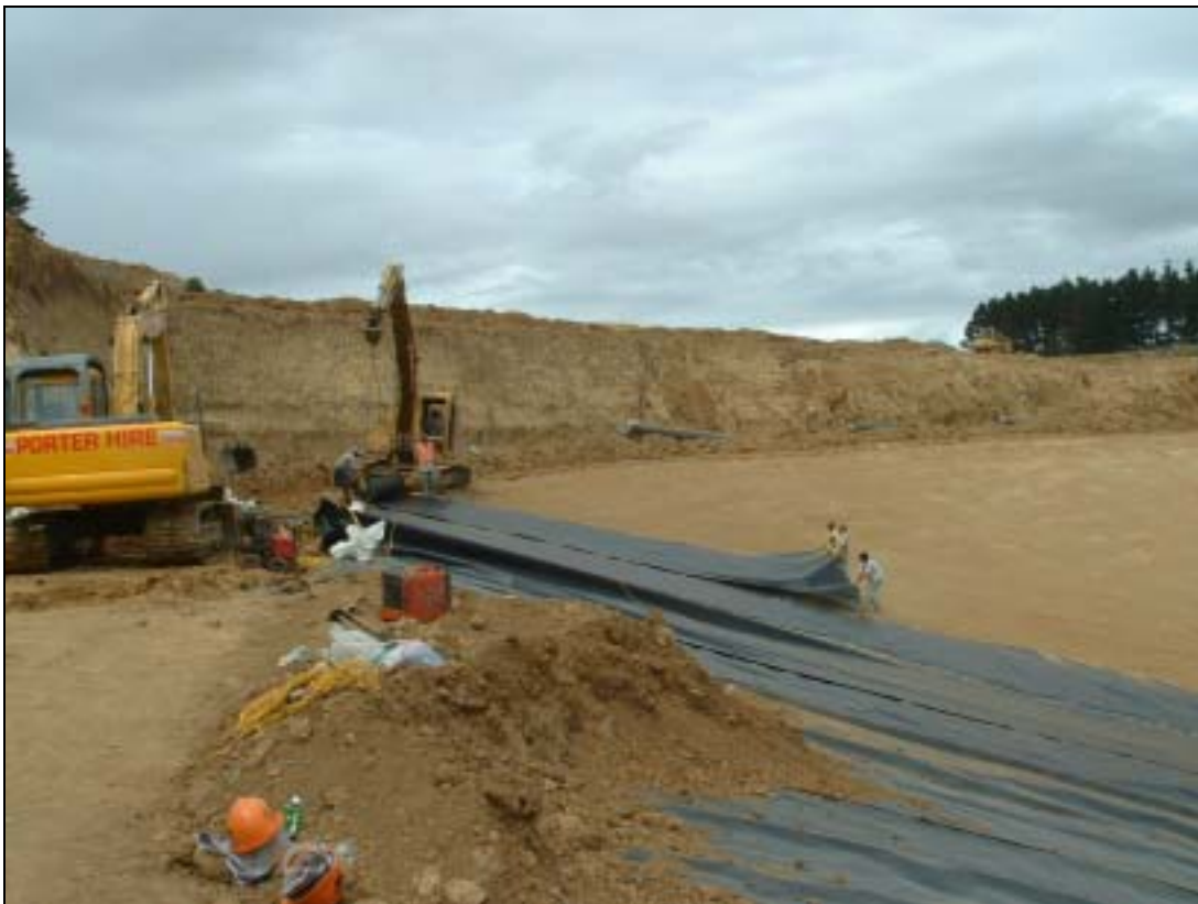
Photograph 1 Laying the HPDE liner in stage three of Colson Rd Landfill, May 2006
