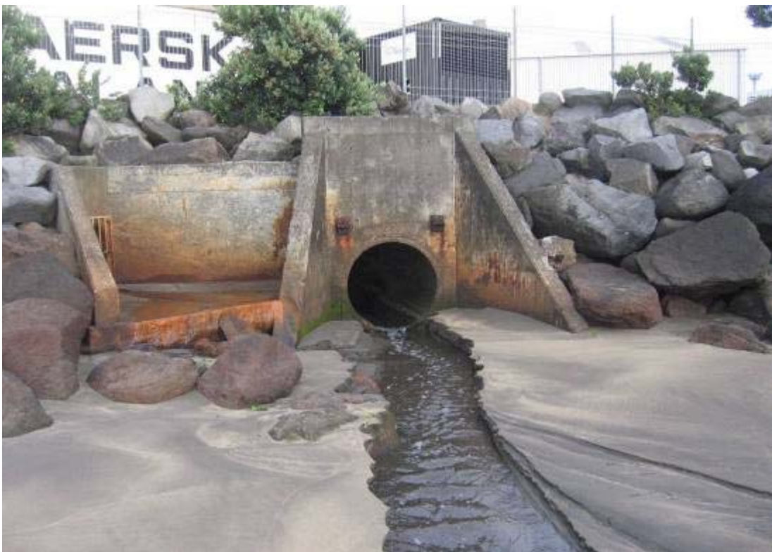
Photograph 6 The Hongihongi Stream enters the western corner of Ngamotu Beach, with a stormwater drain on the left
