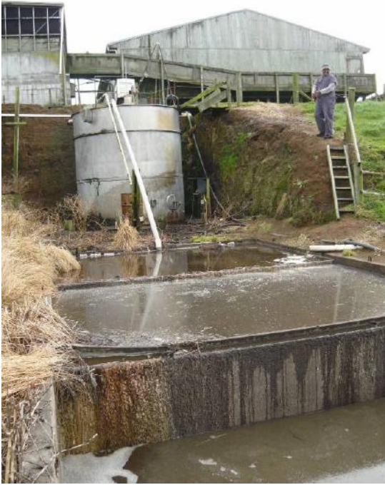
Photo 4 Collection sump and pumps
