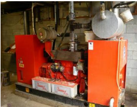
Photo 6 Six cylinder diesel engine and generator
