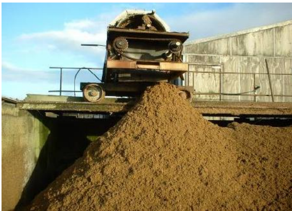
Photo 2 Solids separator and collection system
