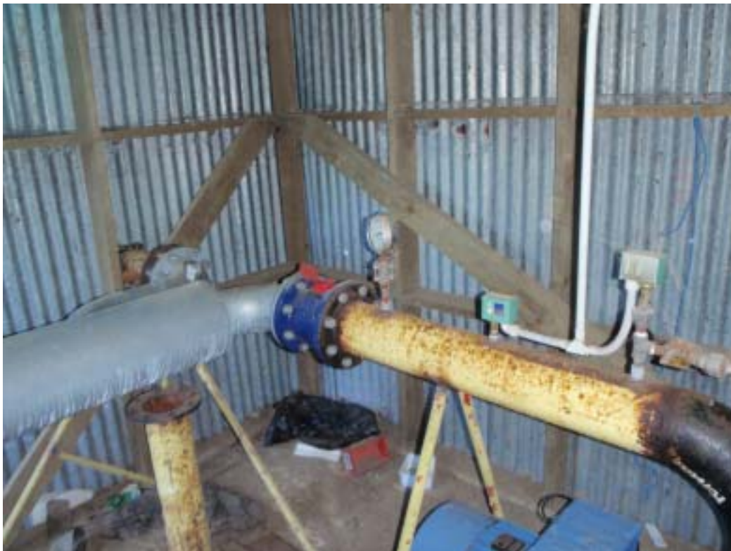
Photo 7 Improperly installed flowmeter
