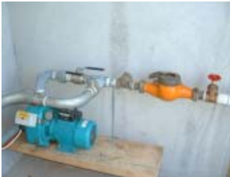
Meter too close to control valves, T and in only one branch of distribution pipes
