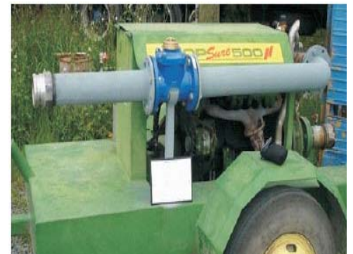
Flowmeter installation in a mobile pump
