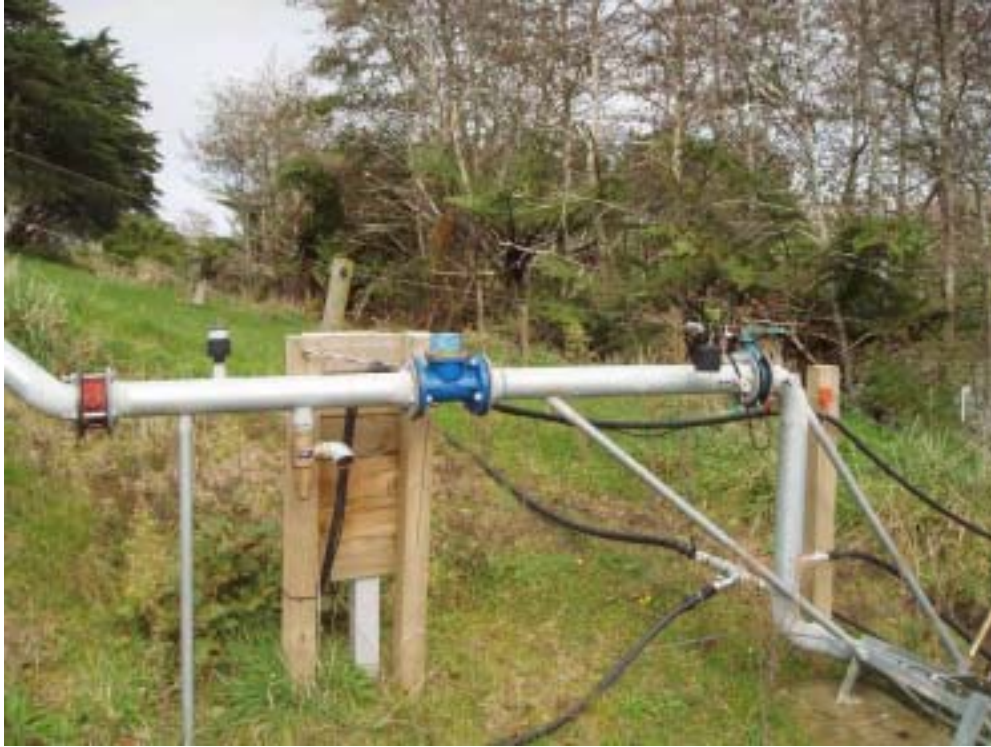
Photo 6 Properly installed flowmeter
