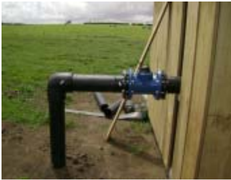
Meter too close to elbow
