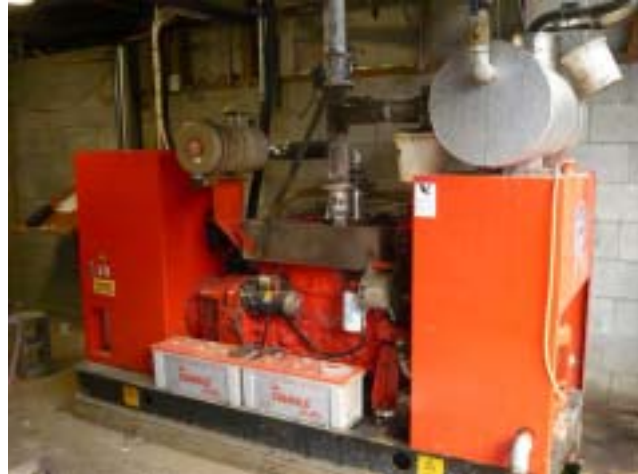
Photo 6 Six cylinder diesel engine and generator
