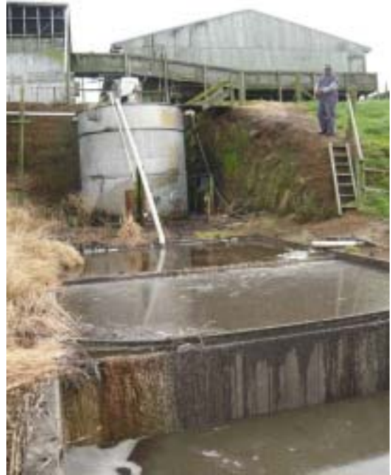
Photo 3 Collection sump and pumps
