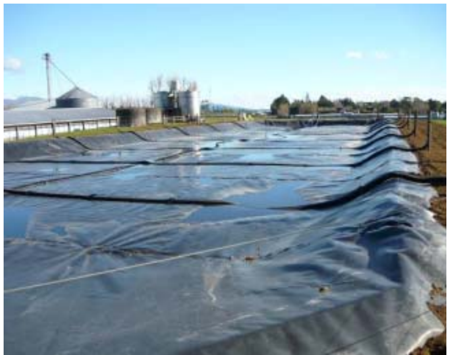
Photo 4 Covered anaerobic pond – flexible drainage pipes hold the cover in situ
