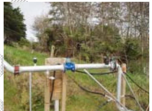
Good installation, sufficient straight length of pip between flowmeter and fittings and bends
