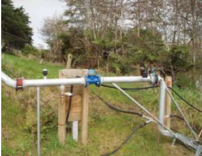
Photo 6 Properly installed flowmeter
