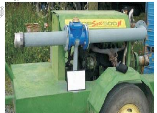
Flowmeter installation in a mobile pump
