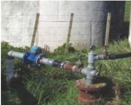
Meter too close to elbow, gate valve and insufficient straight length of pipe
