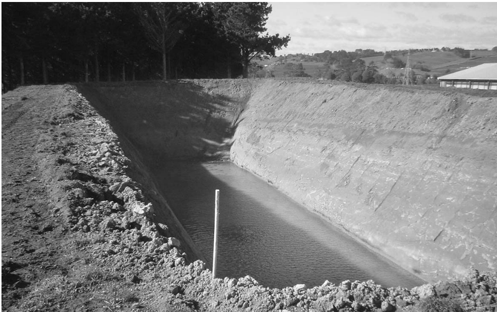
Photo 3 New anaerobic pond
