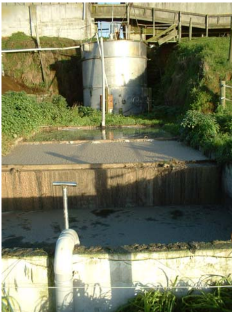
Photo 2 Raw effluent wastewater collection and pumping system
