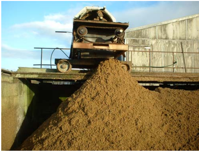
Photo 1 Solids separation and collection system
