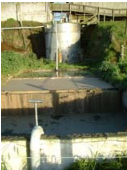
Photo 2 Raw effluent wastewater collection and pumping system
