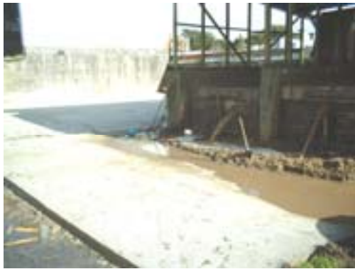
Photo 1 Concrete pad in front of solids separator.
