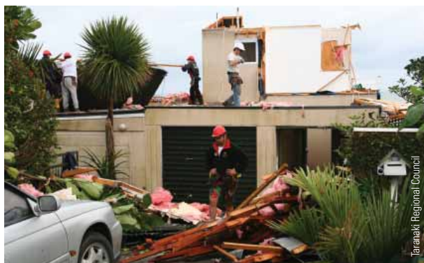
Clean-up operations after the 5 July tornado hit Ōākura.
