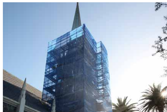
Screens enclose St Andrews Church spire in New Plymouth during restoration work.
